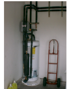
The Heliodyne external heat exchanger heats the domestic water in the unwired electric hot water tank via thermo-siphoning. The heating loop is a glycol/water mix, under modest pressure, circulated with a solar energized DC pump next to the roof-top collector.
