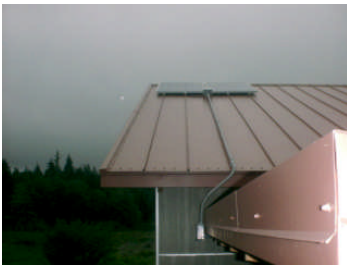
The 360 Watt PV system is modest, for sure, but this weekend cabin is happy, for it is supplied by a 10 KWh sealed battery bank through an Outback inverter.
