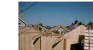
This 12 x 16 SIP (Structural Insulated Panel) building is very energy efficient and useful. The panels were made in Port Angeles.
