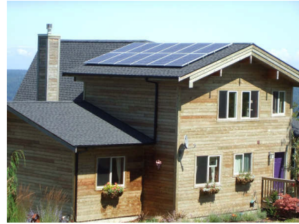
Sequim Bay can be seen in the background of this grid-tied solar electric system. The Evergreen 190 Watt Spruce Line PV Panels work quite well.
